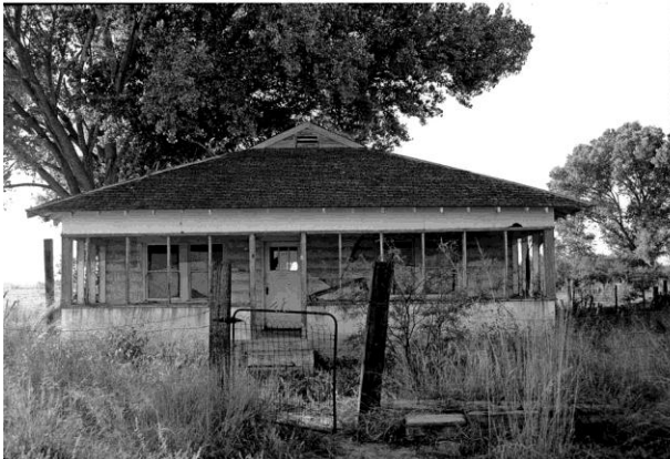
Photo 1. San Pedro House before restoration by Friends of the San Pedro River. BLM Photo
