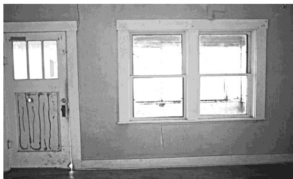
Photo 7. Inside San Pedro House before restoration. Front room showing at right area where sales counter is installed. Note the cracked walls & the hole gnawed in the bottom of the door. BLM Photo
